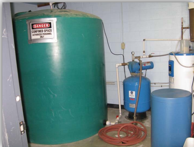
Rollo McClay Water Cistern
