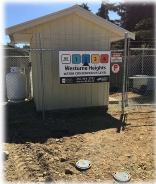
Westurne Heights Pumphouse and Buried Cisterns
