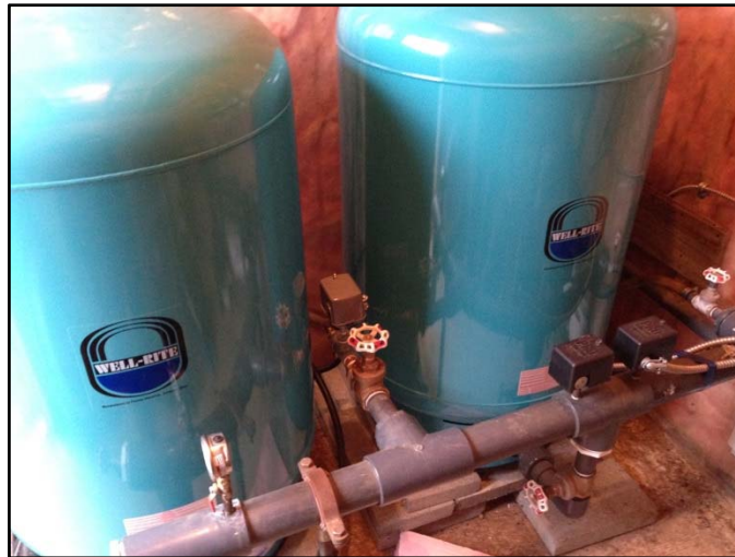
Pressure tanks in the pump house
