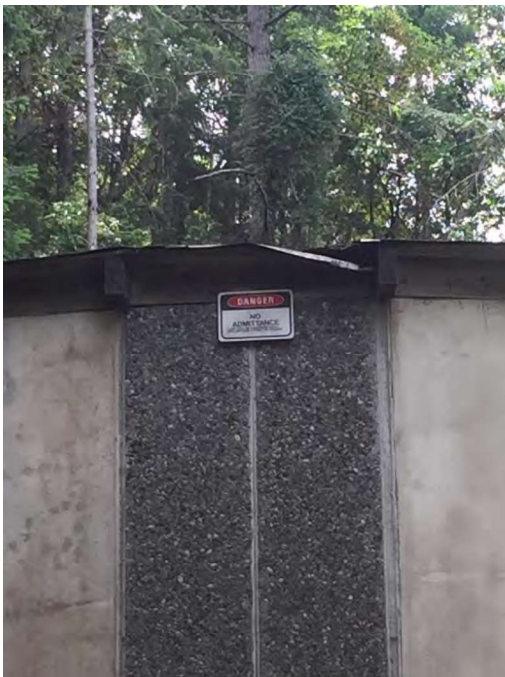
Roof Overhang Damage from 2018 Windstorm
