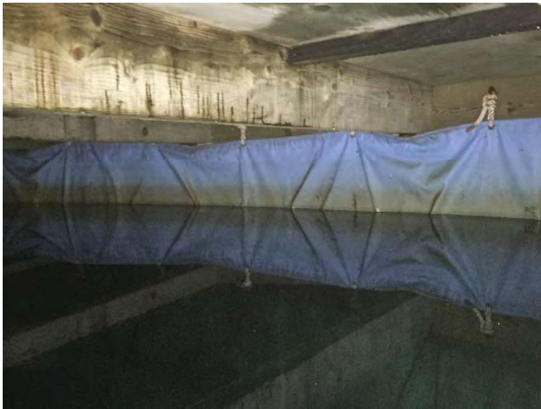
Interior showing bag liner, wood roof joists, and underside of wood roof
