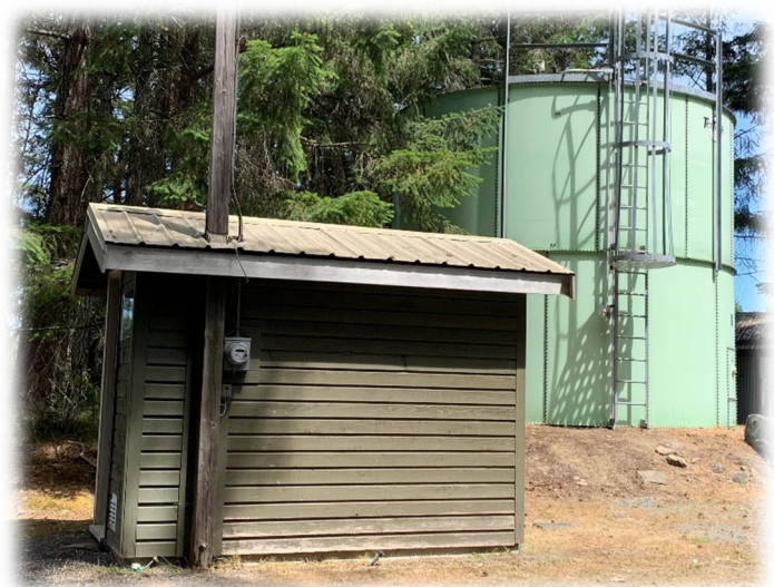
Decourcey Pumphouse and Water Storage Reservoir
