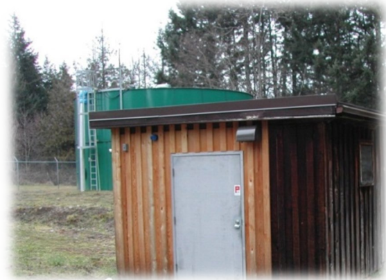
French Creek Main Pump House and Reservoir
