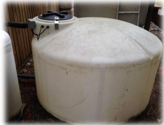
Summer water storage tank at Horne Lake Regional Park
