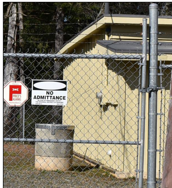
Melrose Well and Pumphouse
