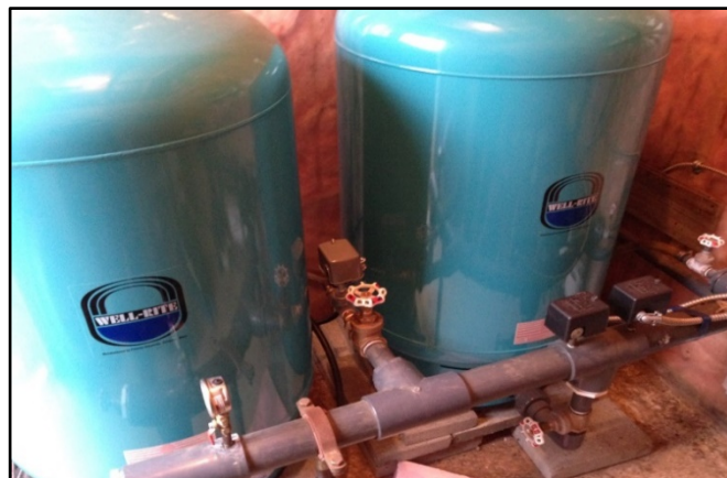
Pressure tanks in the pump house
